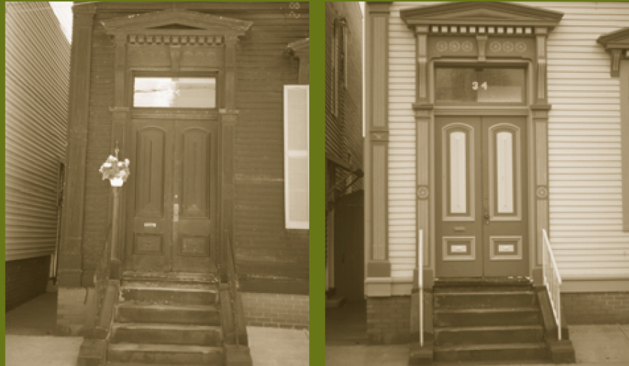
In Restoration , reinstating the historic paint colours from the restoration period should be based on physical or documentary evidence, such as on-site paint analysis and colour photographs.
