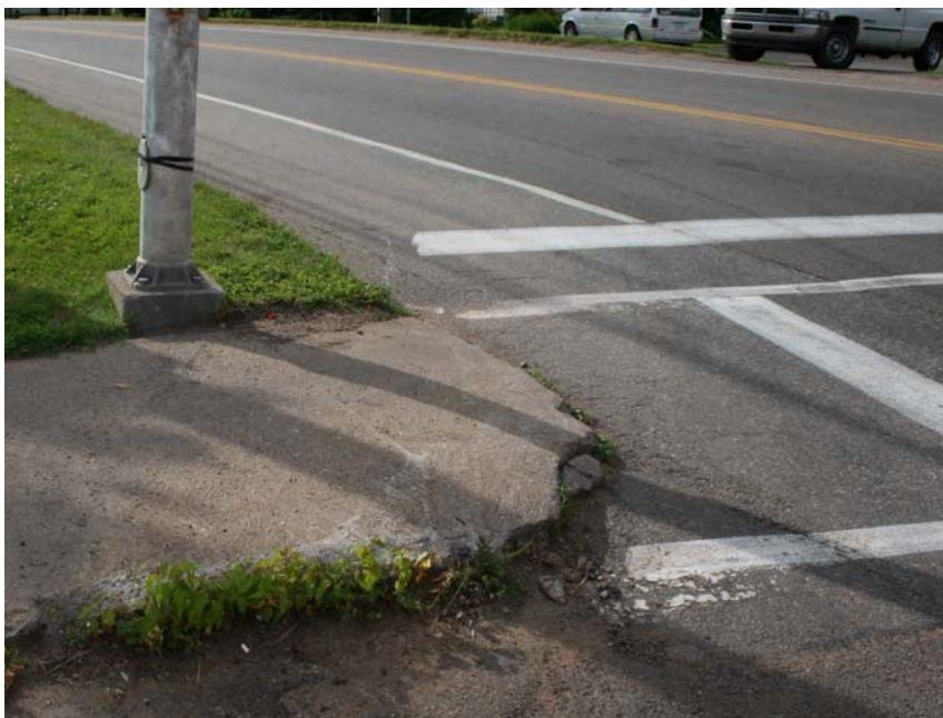
This curb radius is very small and likely causes drivers to mount the sidewalk—a hazard for pedestrians. In this location there is no curb ramp, making it very difficult to traverse for wheelchairs, walkers, strollers and so forth. (McCormick Rankin Corporation)
