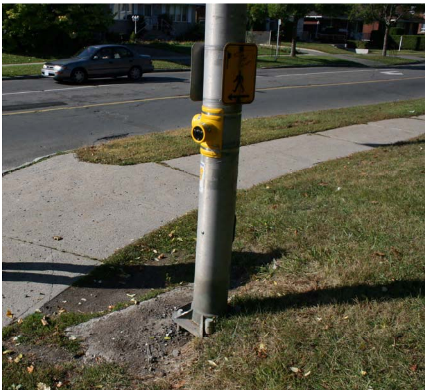
Supplementary information signs and accessible push buttons (for special needs users) can assist pedestrians. This is an example of a deteriorated push button sign that is poorly located. It would be very difficult for a mobility challenged pedestrian to use this push button—particularly during the winter months. (McCormick Rankin Corporation)
