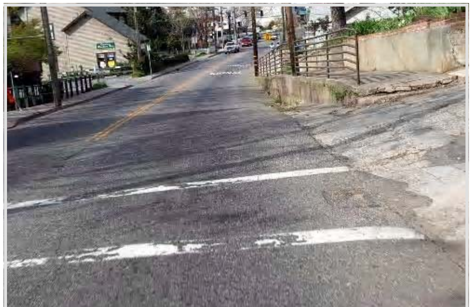
This photo illustrates a poorly marked, narrow crosswalk on a steep slope. In addition, there doesn't appear to be an adequate pedestrian refuge at the end of the crosswalk. (www.pedbikeimages.org / Dan Burden)
