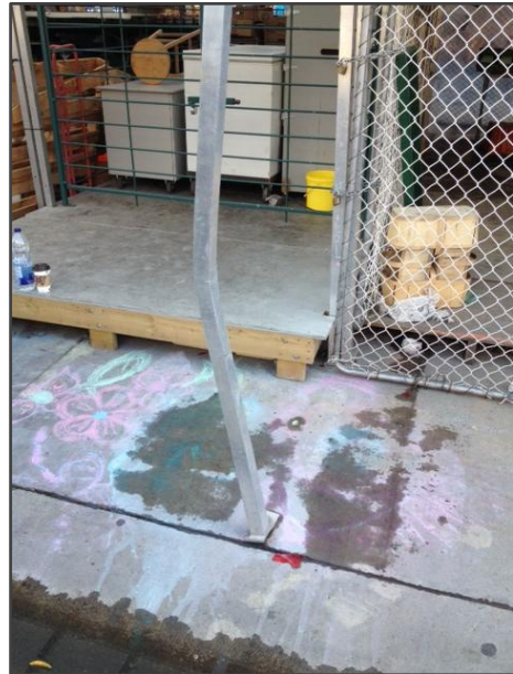
Vendor stand damage due to car collision over night; such damage is frequently reported and/or repaired by Ambassadors.
